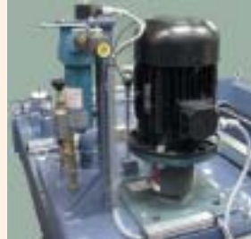
High-Pressure Pump Package
