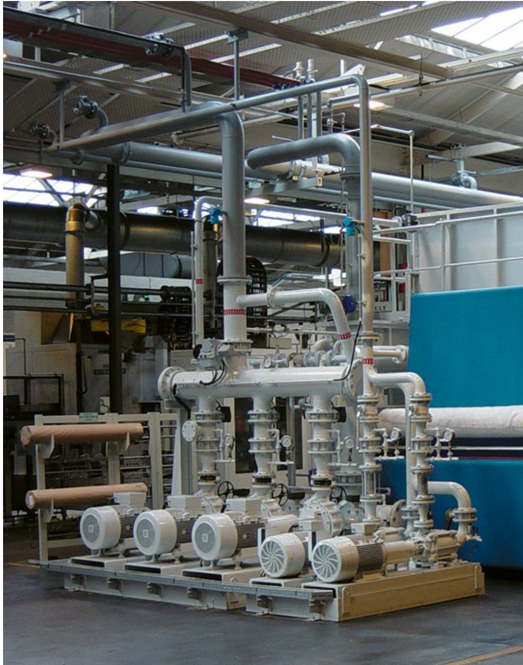
Vacuum filter facility with Viavent pump system
