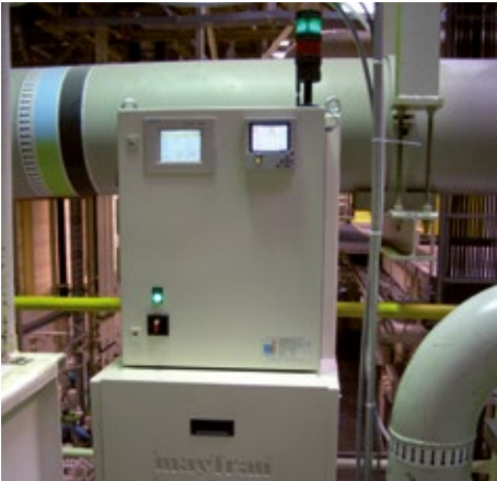
RefillMatic control unit
